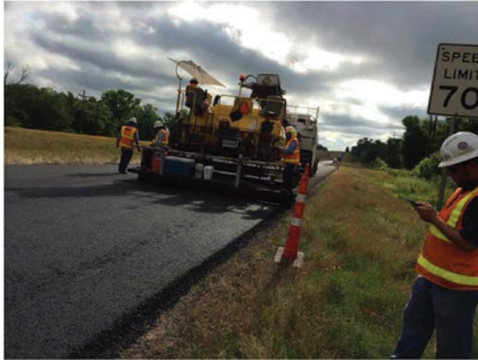
Figure A.11: Mix with Higher Production Temperature Placed beyond Speed Limit Sign.
