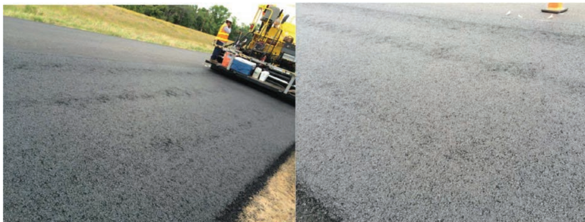
Figure A.10: Segregation behind the Paver—Section 4.
