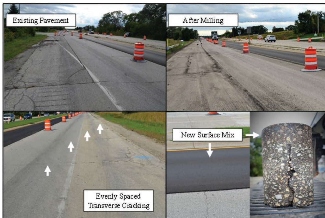
Figure D.2: Existing Pavement Condition.
