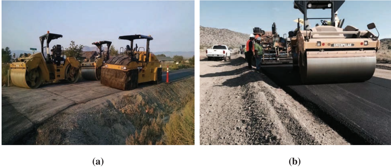
Figure B.6: Picture of (a) Fleet of compactors; and (b) Breakdown roller behind the paver.
